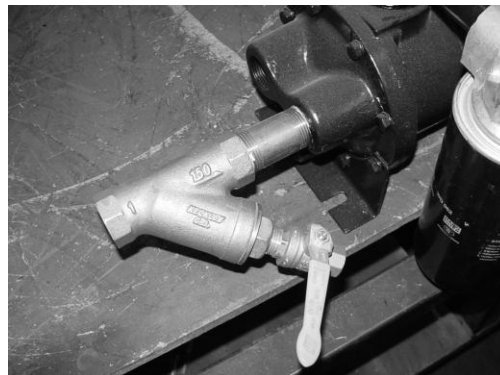
Figure 4 Wye-strainer installed, with cleanout valve.
