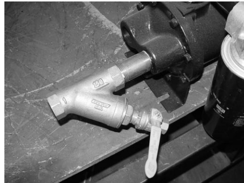
Figure 4 Wye-strainer installed, with cleanout valve
