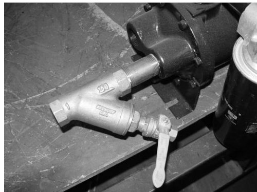
Figure 3 Wye-strainer installed, with cleanout valve.
