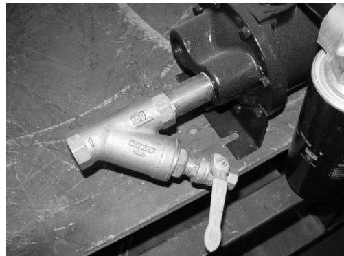
Figure 5 Wye-strainer installed, with cleanout valve.
