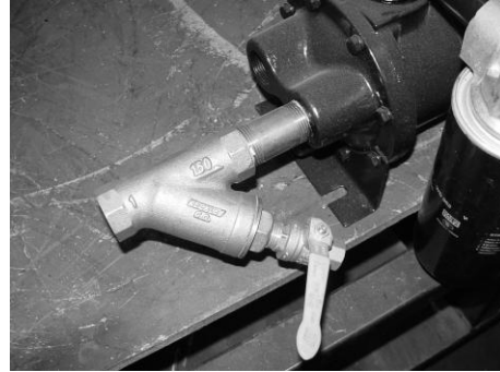
Figure 5 Wye-strainer installed, with cleanout valve.
