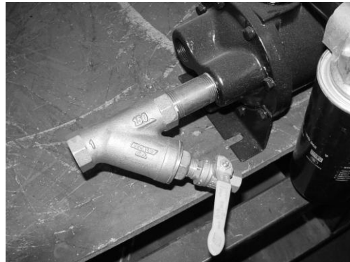
Figure 4 Wye-strainer installed, with cleanout valve.
