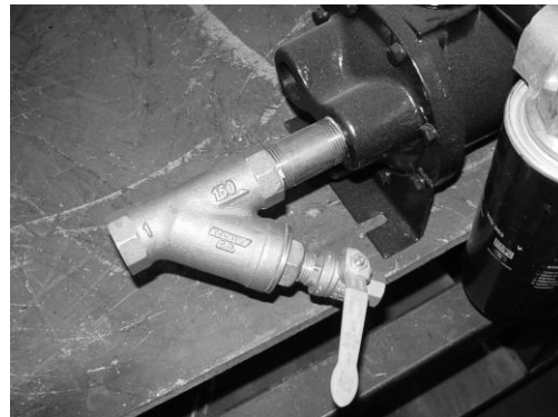
Figure 4 Wye-strainer installed, with cleanout valve.
