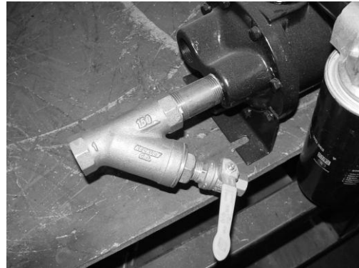
Figure 3 Wye-strainer installed, with cleanout valve.
