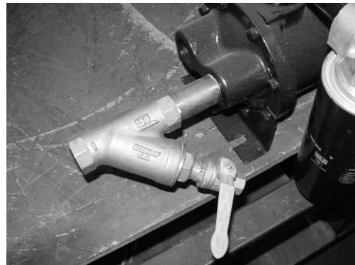
Figure 4 Wye-strainer installed, with cleanout valve.
