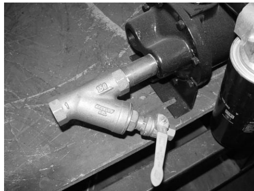
Figure 5 Wye-strainer installed, with cleanout valve.
